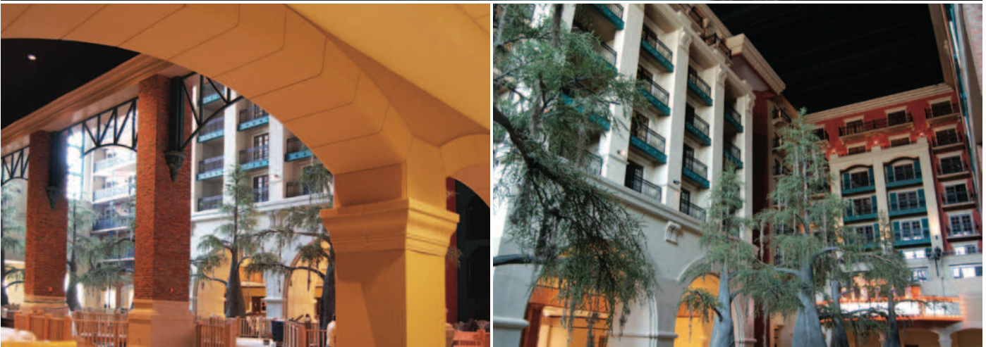
Fiberglass Ornamentation for entire atrium interior, buildings, trim and facades, Paragon Casino Resort atrium complex, Marksville, LA
